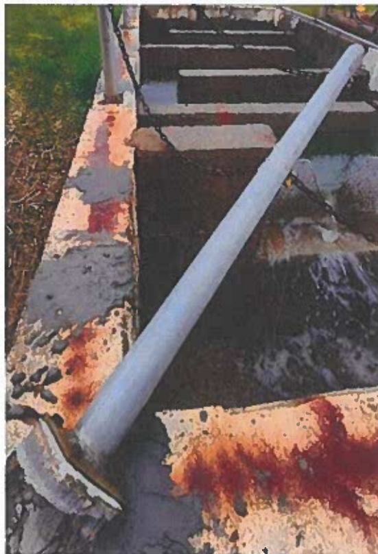
Photo 4: Water seeping around v-notch weir plate and recent concrete repairs with broken post.
